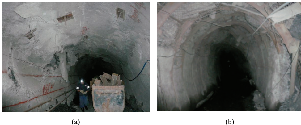
Fig. 3. Actual deformation of surrounding rock and deep roadway section: a – the original roadway section, b – deformation of roadway surrounding rock
